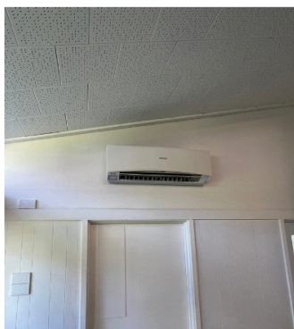
Heat pump in main coworking space
