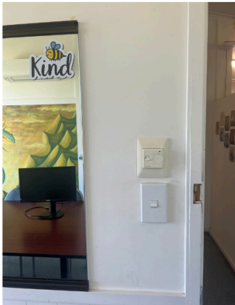
Meeting Room 1 roof heaters
