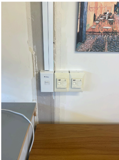
Other light switches & wall heaters for coworking space
