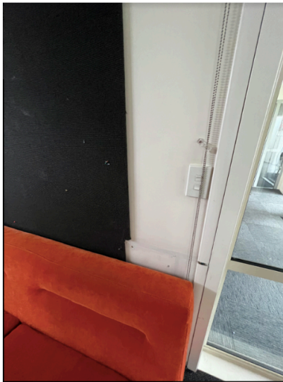
This lightswitch turns on the lights for the corridor and adjacent rooms in the lunch room and end meeting rooms (3,4)
