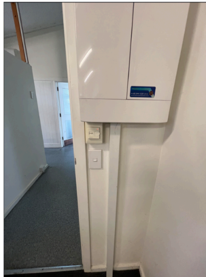
Find the light switch for the main coworking space here.
