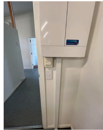
Coworking space roof heaters
